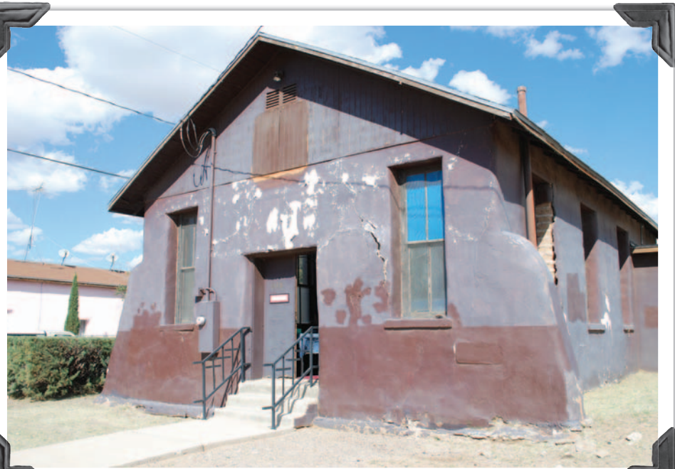
Before restoration began, obvious cracks could be seen in the façade of Phillips Chapel. Even more damage was discovered behind the plaster covering the adobe walls.
