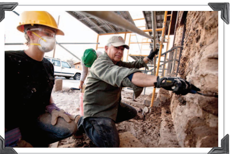
Course instructor David Chavez explains to Stephanie Sweet the process of adding adobe to the building during a student workday in February 2011. That was the last semester the DACC preservation class was held.
