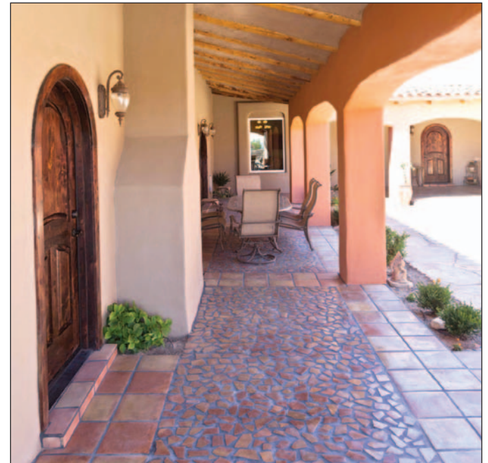
Broken Saltillo tile lines the covered patio.
