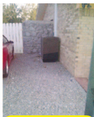
Completed 5 Ton System
