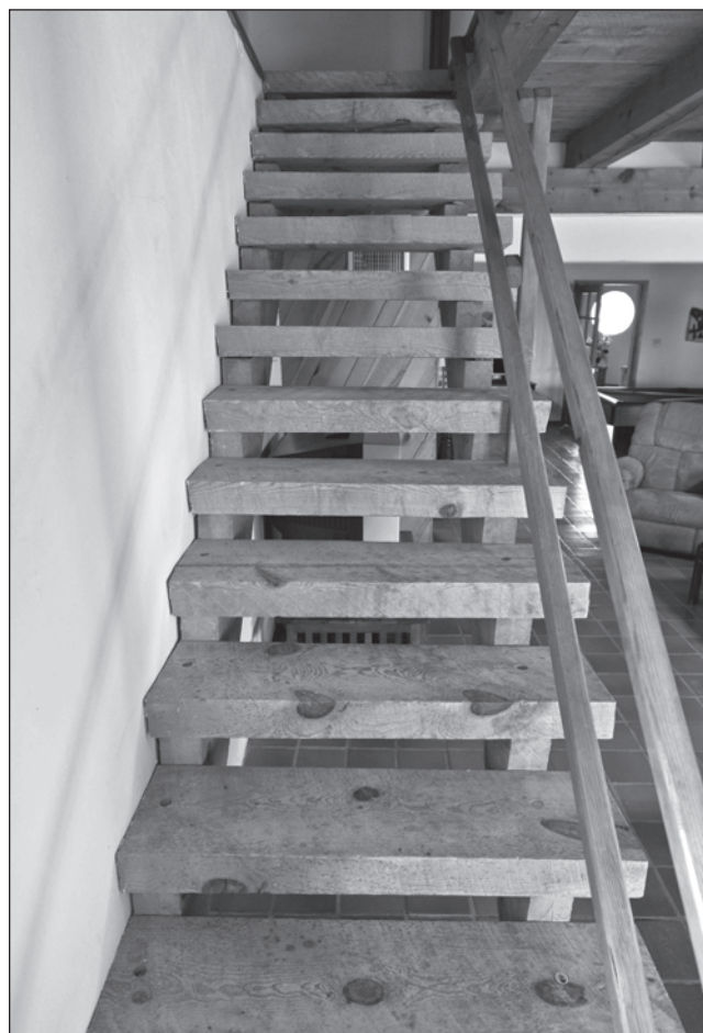
Stairs lead to the second floor, which was part of a 2,500-square-foot addition to the home.
