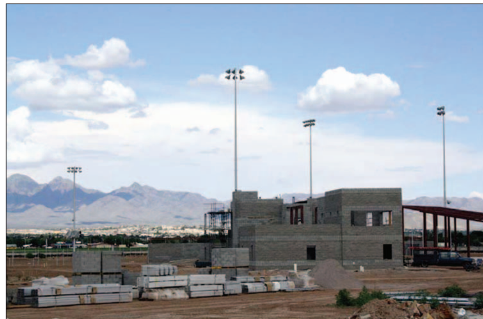
Stands for the new Las Cruces Public Schools' baseball fields on Tashiro Road, south of the Field of Dreams football stadium, is taking shape. The project is expected to be complete in time for the 2013 high school baseball season in February 2013.
