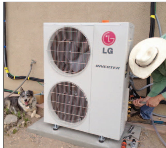
Installation of the outdoor unit for one of the ductless mini-split systems in the Dyson home.
