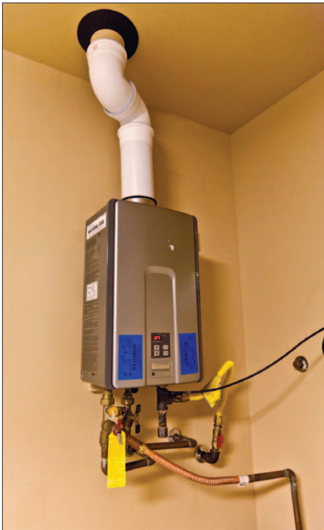
A tankless-water heater helps with the home's efficiency.
