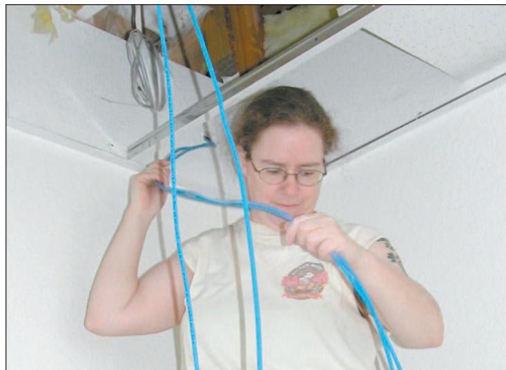
Lynne Happe works on Internet wiring into classrooms of the J. Paul Taylor Academy Tuesday, July 12. The new charter school for elementary-age students opens its doors Monday, July 25, at 3900 Del Rey Blvd., a former pre-school building. An open house will be held at the school from 2 to 4 p.m. Saturday, July 23.
