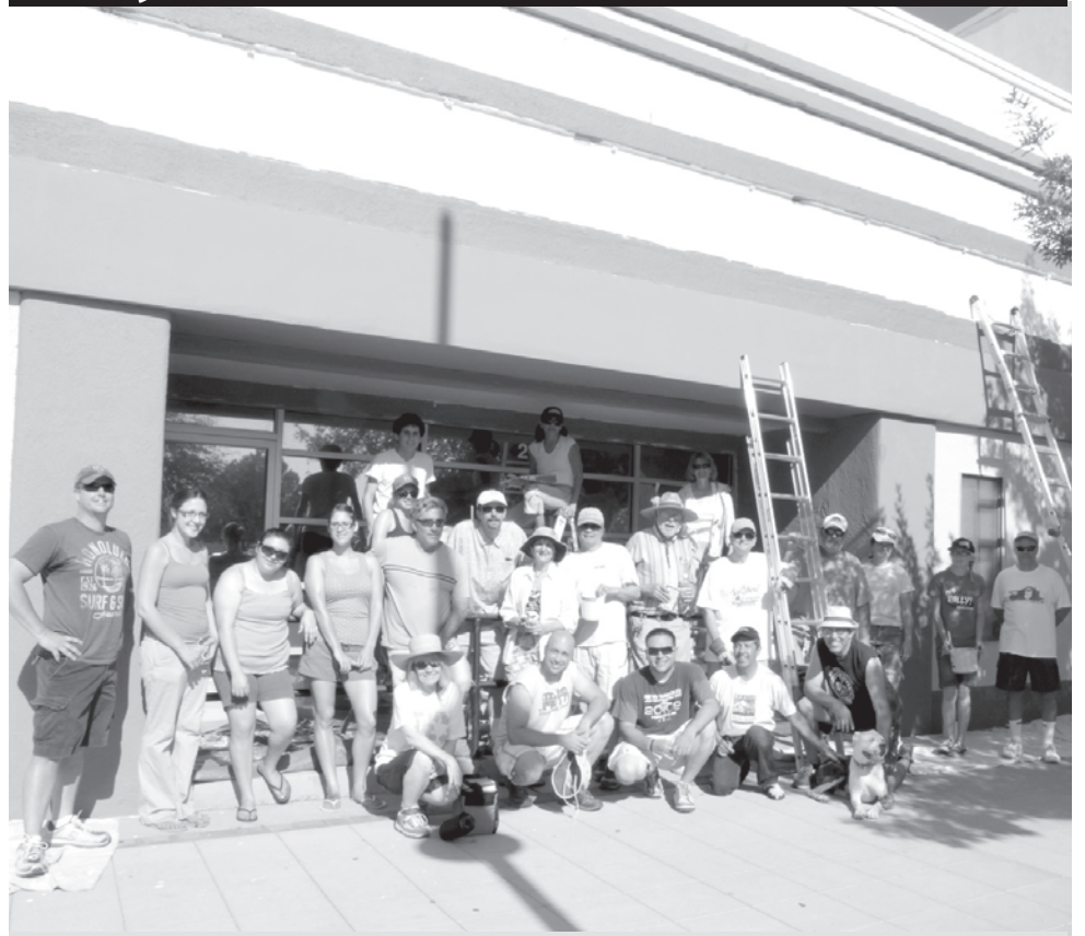
More than 30 volunteers braved the summer heat to repaint three Downtown properties in Las Cruces as part of the Downtown Las Cruces Partnership's Façade Squad initiative, which took place during three weekends in June and July.
