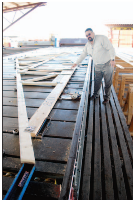
Jack Herndon of L & P explains how all of the trusses are created at the facility.
