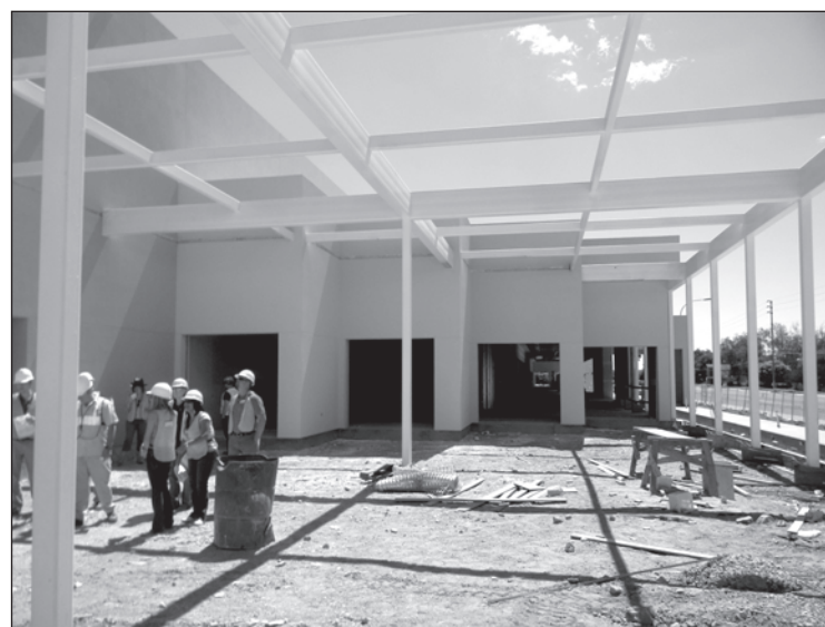
While under construction, Las Cruces Convention Center crew members stuck to a strict plan to make the building as green as possible. The work paid off and the convention center has been awarded LEED Gold status by the U.S. Green Building Council.
