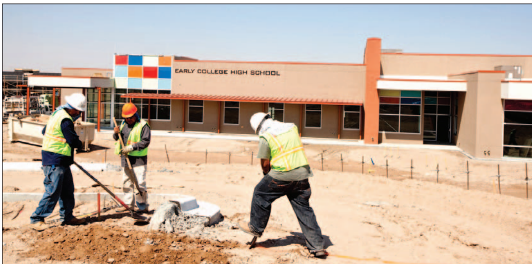
A crew prepares to set down cement Tuesday, June 7, at the Arrowhead Park Early College High School on the New Mexico State University campus.
