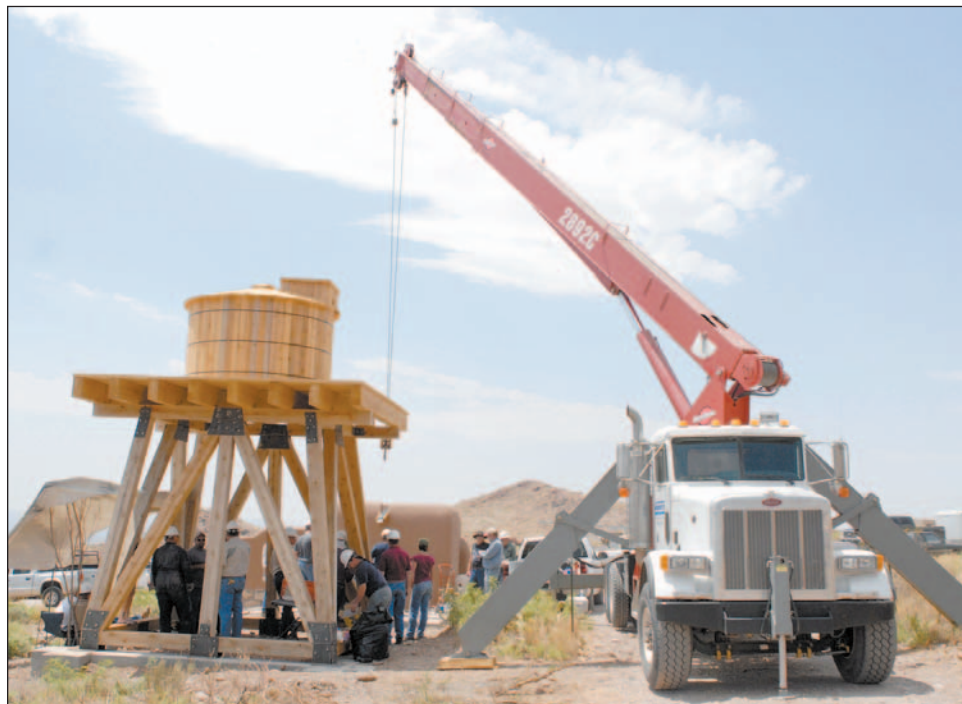
A crane lends a helping hand while installing a 27-foot-tall windmill with 10-foot blades that will be used to draw water on the property of Wayne and Elizabeth Grinnell at 12520 Canyon de Oro Friday, June 3.
