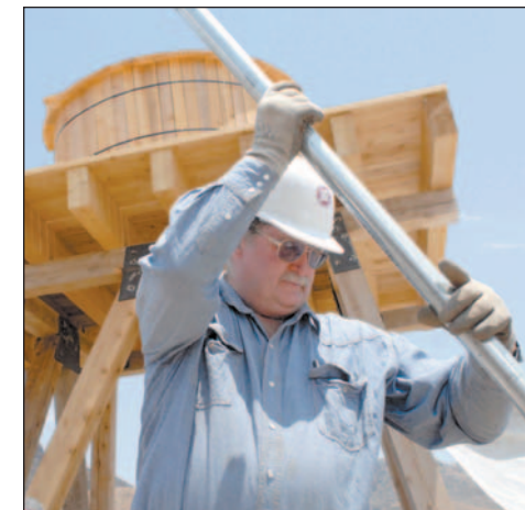
Philip Leiendecker from Arizona helps out while installing a new 27-foot-tall windmill made to draw water from a well to an adjacent wood water tower. Leiendecker is part of a three-day workshop on windmill repairs and installation held by New Mexico State University.
