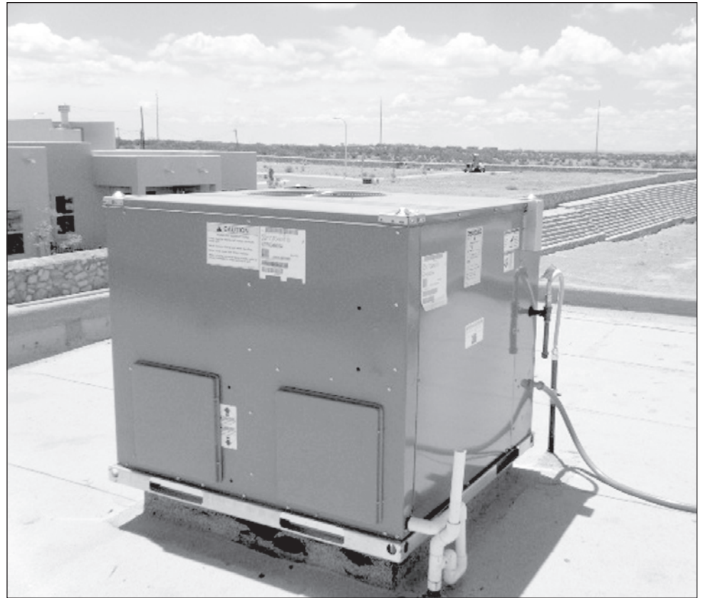
Stay cool this summer by properly maintaining your rooftop mounted package air conditioner and gas heating unit.
