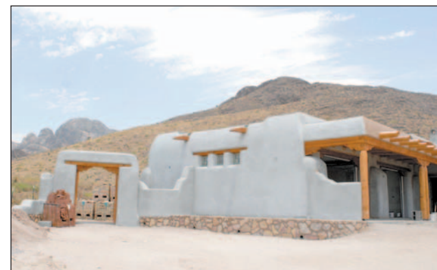
The Grinnell home is currently under construction by Classic New Mexico Homes.
