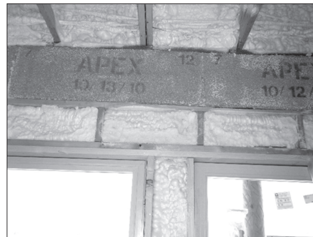
Insulated concrete form walls combined with spray foam insulation fill the attic and wall sections in this David Coyle Home currently under construction and targeting Build Green New Mexico gold certifications in Las Cruces.
