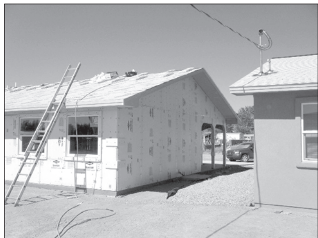
The Otero County Habitat for Humanity used rigid insulation installed at the exterior walls of a home, which was built to Build Green New Mexico silver certification in Tularosa.
