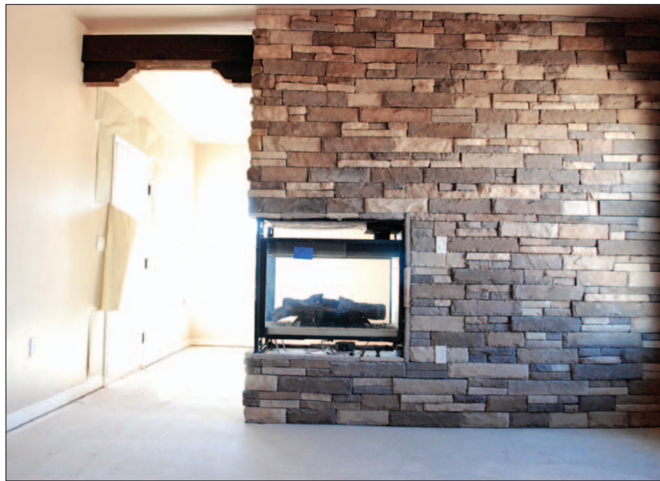
Also currently under construction, Benavidez included a three-way fireplace to divide the space in the master suite between the bedroom area and at-home office.
