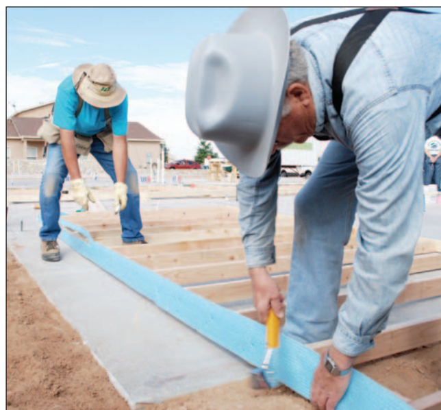
Local volunteer Bob Lytle and MVHFH Construction Superintendent Don Stover work on the first of six homes completed during the 2010-11 build season.
