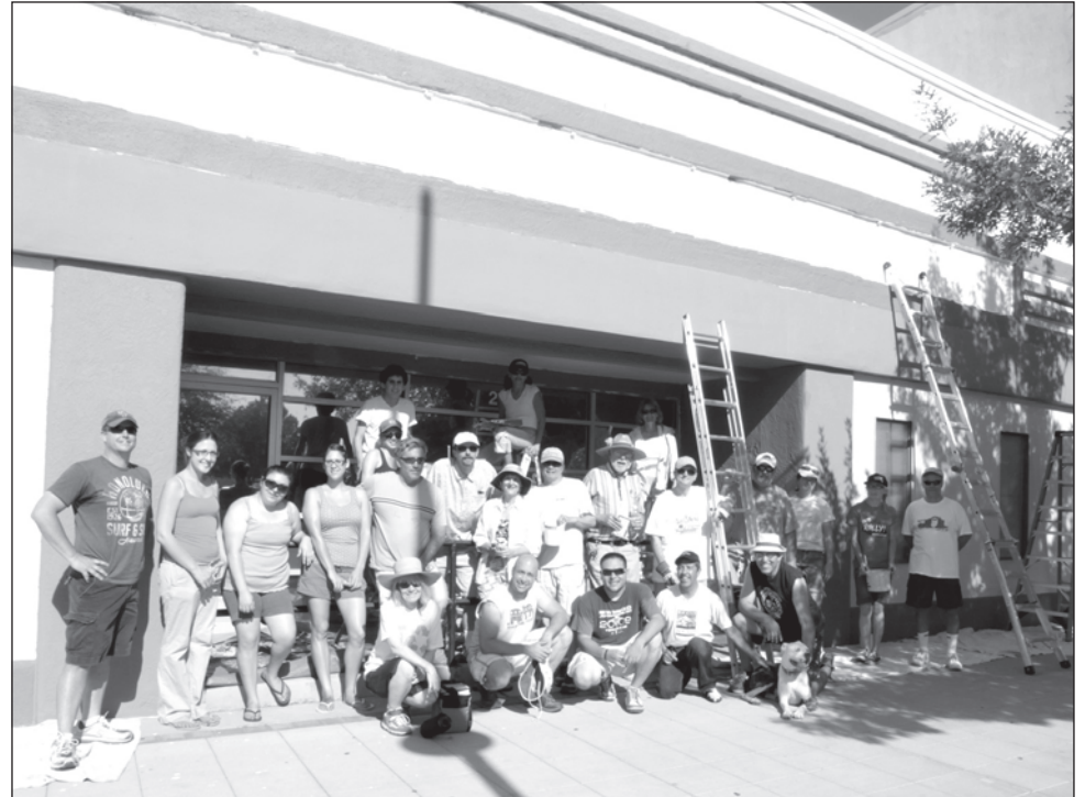
More than 30 volunteers braved the summer heat to repaint three Downtown properties in Las Cruces as part of the Downtown Las Cruces Partnership's Façade Squad initiative, which took place during three weekends in June and July 2011.
