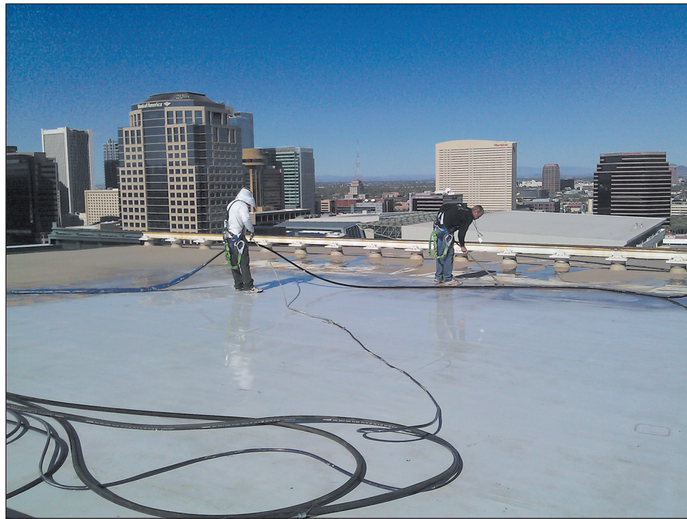
Farrell Thurston has recently introduced elastomeric roofs by the KM Coating Shieldcoat System. The company, based in Phoenix, uses the material to restore Chase Field, home of the Arizona Diamondbacks.
