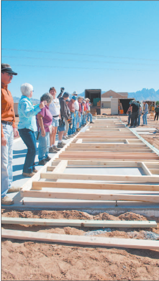
Locals and care-a-vanners prepare to lift the first wall of the first home of the Mesilla Valley Habitat for Humanity 2011-12 build season Monday, Oct. 10, on Calle Bella.
