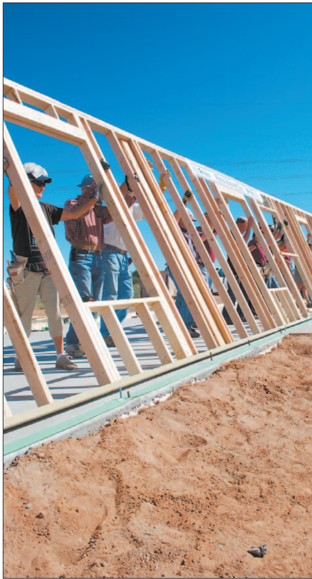
The raising of the first wall marked not only the beginning of the build season, but also honored World Habitat Day.
