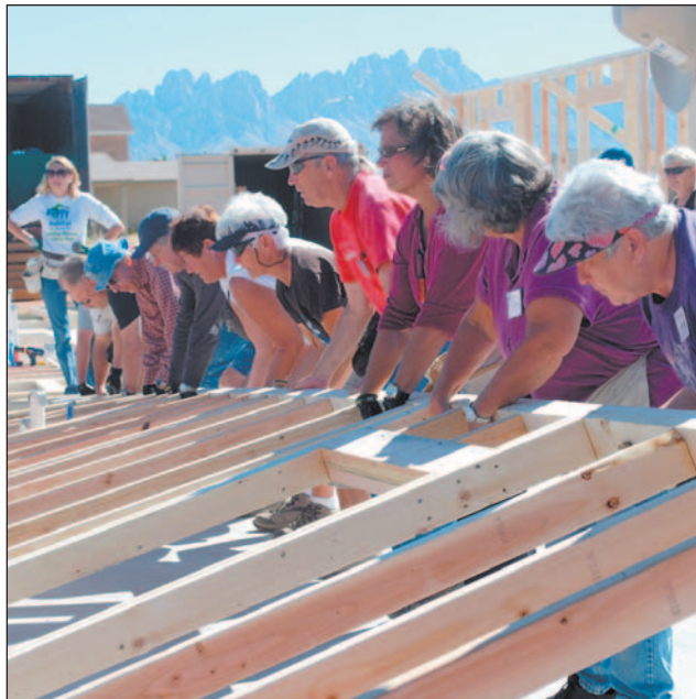
Volunteers move on to lifting the second wall of the four-bedroom home.
