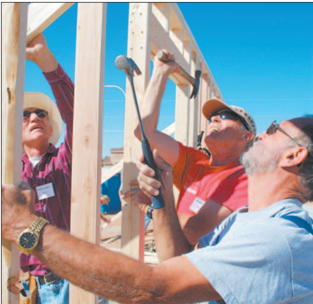
Care-a-vanners Paul Stoutenborough and Bruce Wilson and local Robby Robertson secure the support of the wall.
