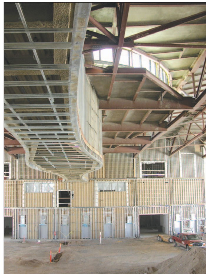
In the center of the building is the 47,000-square-foot hangar, with this third-floor walkway linking the entrance to the exclusive "astronaut's lounge."
