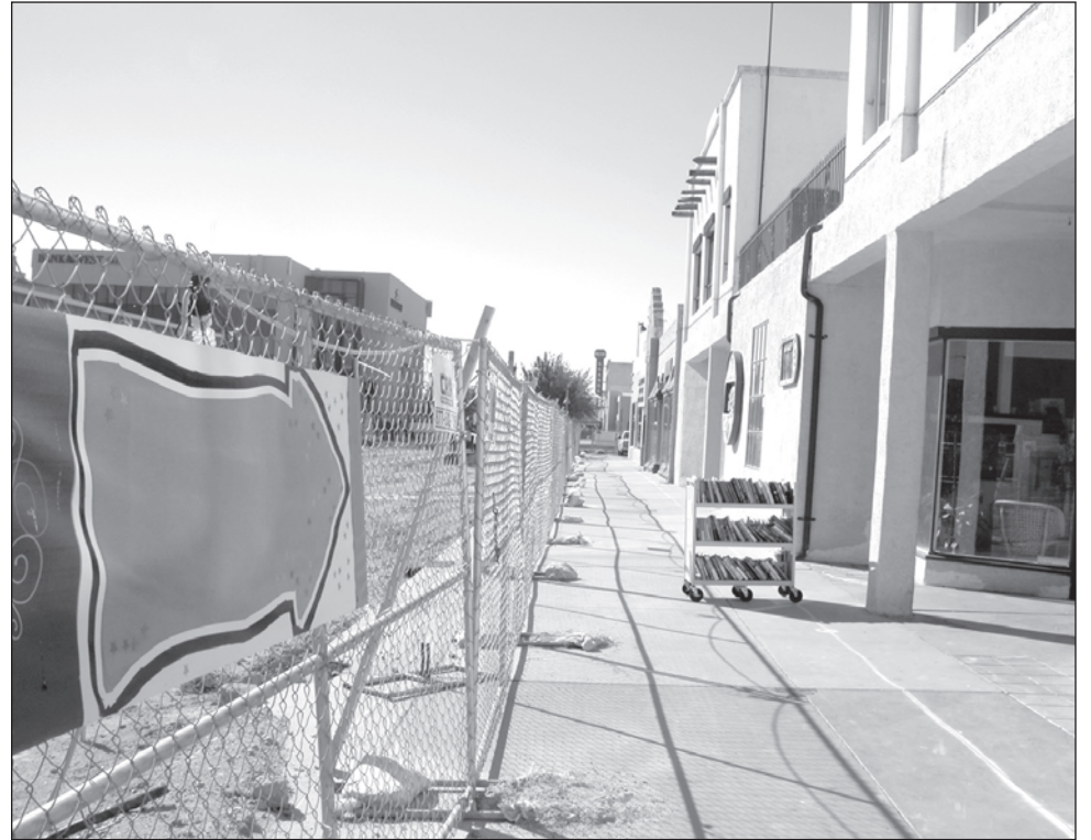
Use the wayfinding arrows painted around Downtown to find your business of choice amid the Main Street renovation construction.
