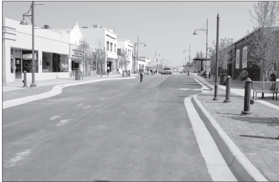
As the fences come down on North Main Street, crisp roads and open store fronts are revealed. Construction on the north end is expected to be completed in October.
