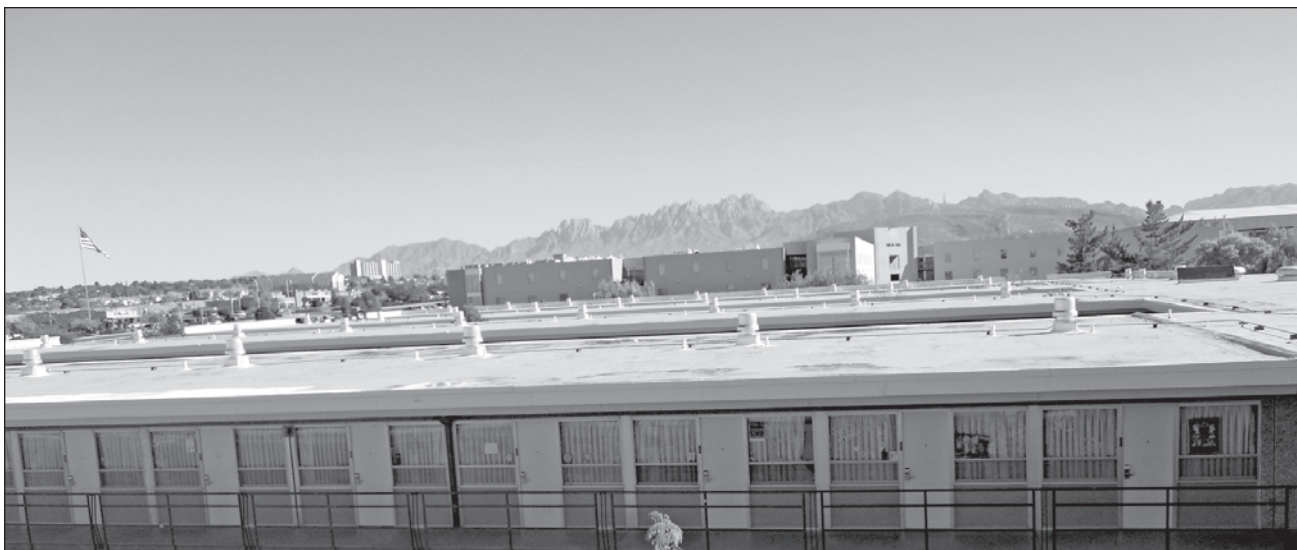
Before the installation of the cool roof system in May, the roof of Garcia Hall was covered in asphalt, which made the building inefficient because it would absorb heat, making the air conditioning units work harder to cool.
