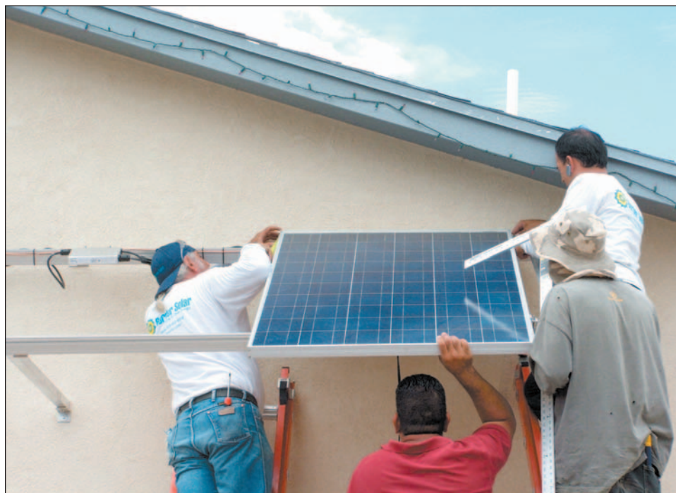
Community members in Anthony, N.M., were trained by Tierra del Sol to install solar panels onto three homes in the community. Solar panels will be included on other homes built by the housing organization, which serves southern New Mexico and west Texas.
