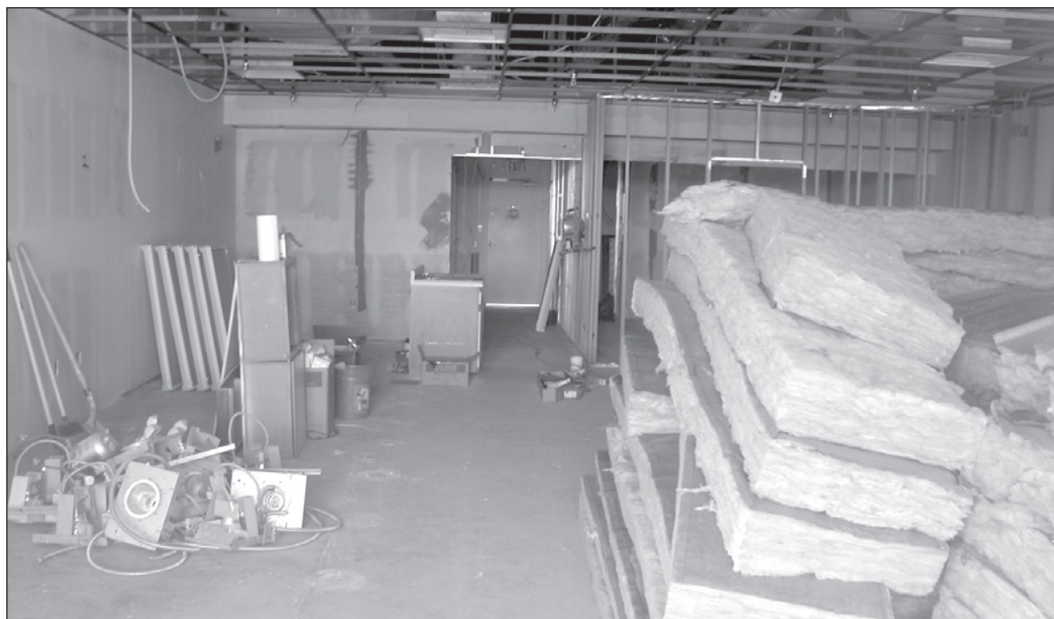
The interior of a Pan Am Plaza retail space is being gutted to make room for the new Okazuri Sushi Bar.
