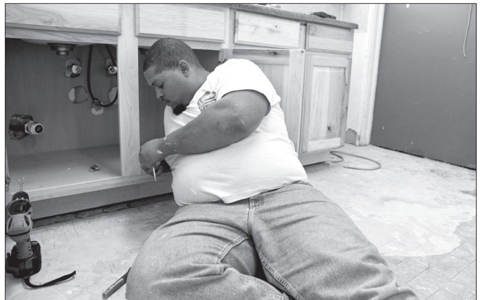
Lowe's Employee Quincy Leake does some cabinetry work at the Boys & Girls Club of Las Cruces.
