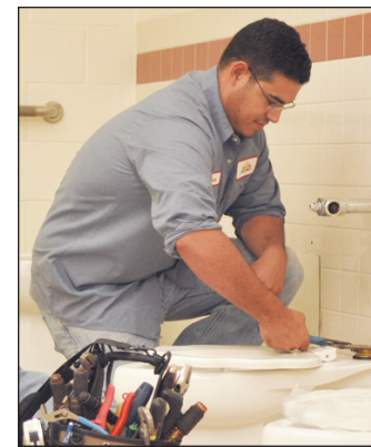
Jason Olguin of Sun City Plumbing and Heating works on installing toilets at the Child Crisis Center.
