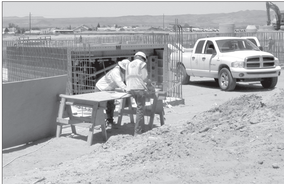
Burn Construction Co. Inc. workers working on the Del Rey/Sandhill Arroyo infrastructure project on Del Rey Boulevard. The project, which aims to add sidewalks, curbs and gutters, drainage structures, storm drains, bike lanes and pedestrian facilities, is part of an American Recovery and Reinvestment Act grant. Jobs created include equipment operators, electricians, carpenters, cement workers, iron workers, truck drivers and laborers. The project is less than 50 percent completed and is expected to be finished by the end of the year.
