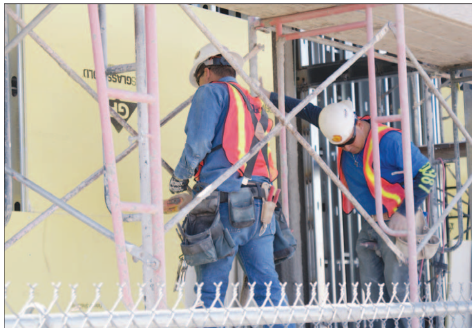
Jaynes Corp. construction workers install panels on the exterior of the Las Cruces Convention Center March 29. The convention center, along with other municipal, state and federal projects, helped the construction industry make modest employment gains locally in 2010. The construction industry lost more than 8,300 jobs in New Mexico in 2009.
