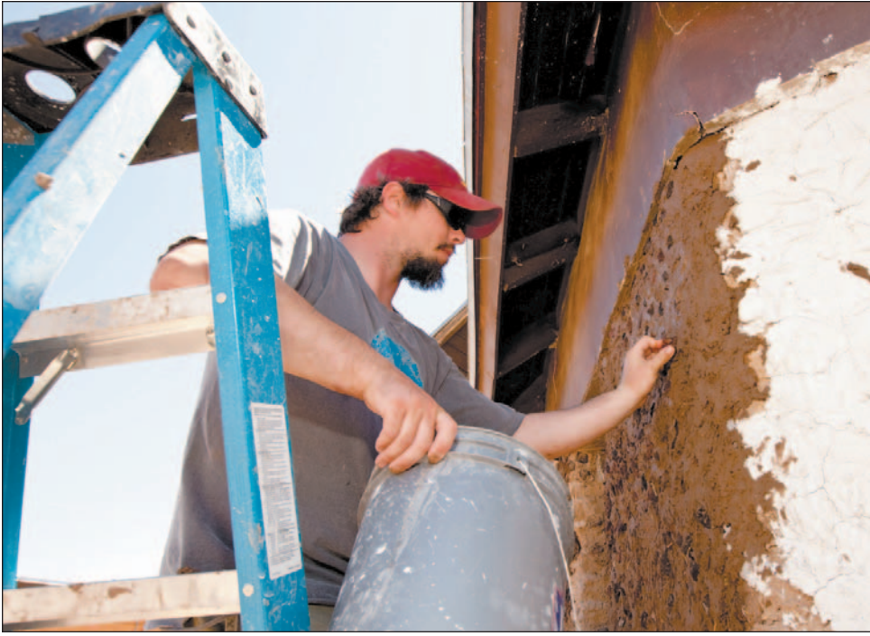
Chad Norred lends a hand to the restoration and conservation project of Phillips Chapel CME Church on Tornillo Street June 19.
