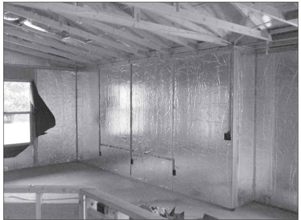
This Silver City Energy Star home is being built by Timberland Construction and uses an inexpensive prefabricated wall system engineered with wood framing at 4-foot centers. The wall sections include rigid high-density insulation to provide R-21 insulating value within an airtight 2-by-4 frame wall cavity.
