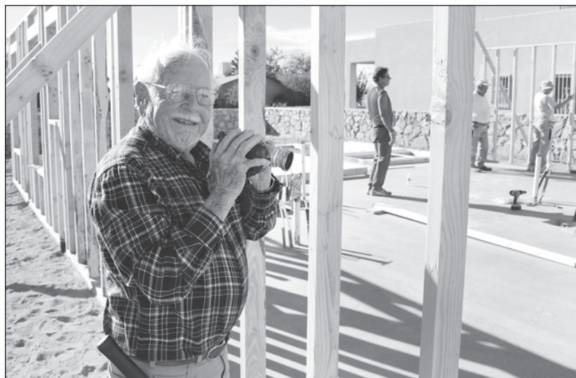
Mac Fell, a volunteer with Mesilla Valley Habitat for Humanity since 1989, videotapes the construction process for homeowners.
