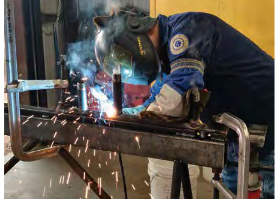
LCU Senior Gas Welder Lupe Valdez welds the new gas line connections for a new customer ensuring high quality work for the LCU gas system.
