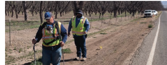
Natural Gas Cathodic Technicians Stephan Klingelmeier and Jesus Roman performing an incremental survey on a gas transmission line by inducing the current to maintain the integrity of the gas system. - Courtesy of LCU
