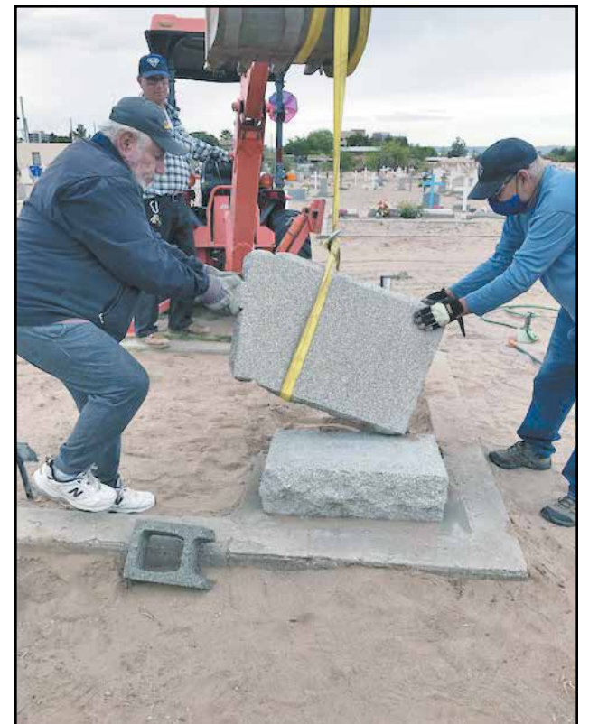
Repairing a headstone at San Jose Cemetery are José Tapia, Jaime Flores and, with the tractor, Paul Alvarado.
