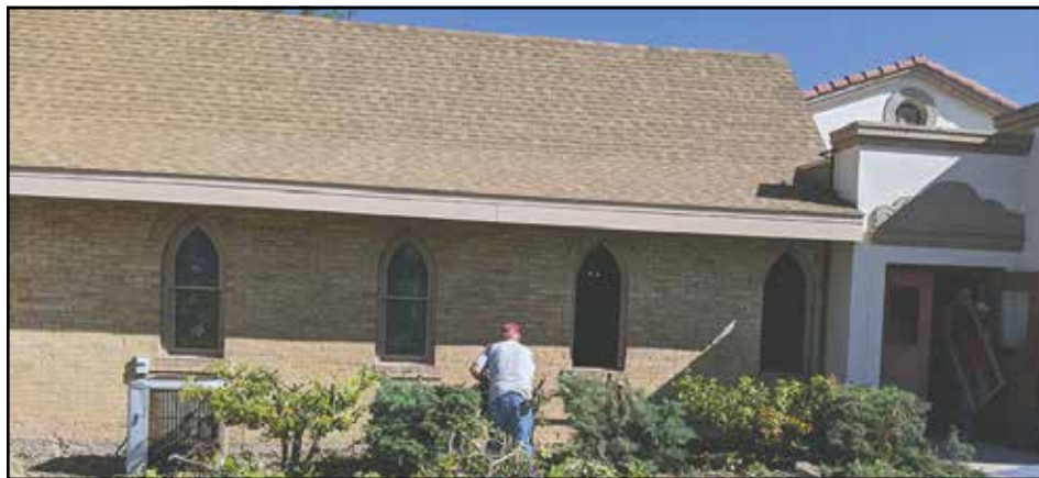
Shrubs were cut down to allow window installations on the south side of Kendrick Chapel.
