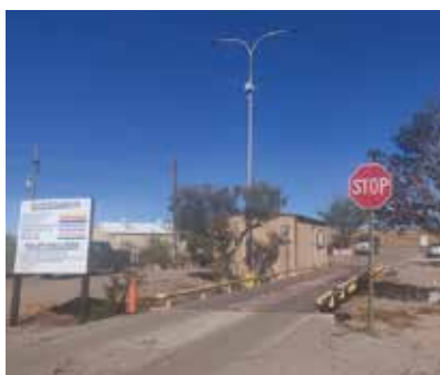
New cameras at the FLCF will help station attendants ensure the loads have no contaminants, instead of needing to climb the trucks to check.
