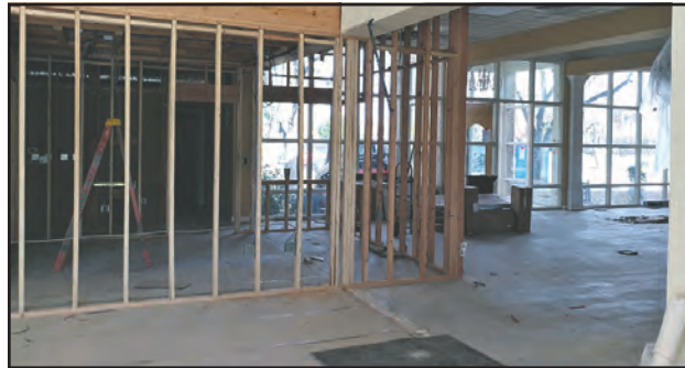
The interior of the Cutter Gallery property as it looked on Dec. 8, as renovation work continued.
