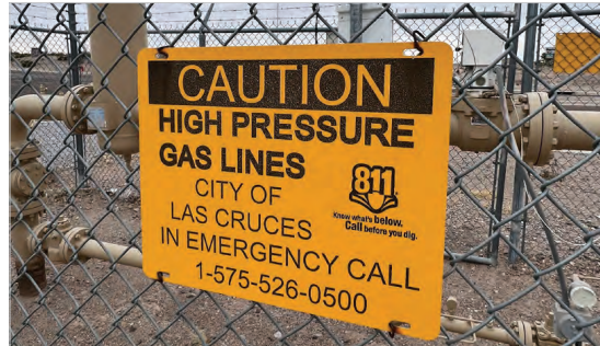
LCU High-Pressure Natural Gas warning sign - Courtesy LCU
