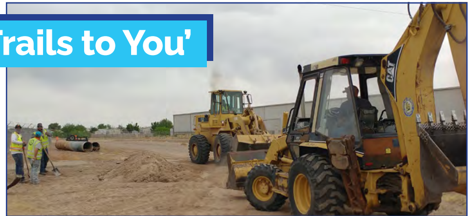
Construction is on-going to finish trails in and around Las Cruces to provide access for healthy walking and activities.
