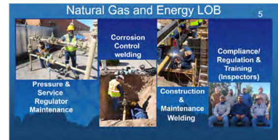
PHOTO 1: LCU Natural Gas and Energy Line of Business slide - Courtesy LCU
