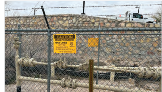
PHOTO 1: Regulator Station - Courtesy LCU
