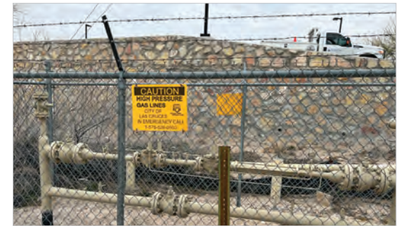
PHOTO 1: Regulator Station - Courtesy LCU
