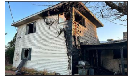
COURTESY OF CITY OF LAS CRUCES A two-story residence in the 2200 block of Desert Drive is seen following a fire that was active on both floors plus the attic on the morning of Dec. 21.
