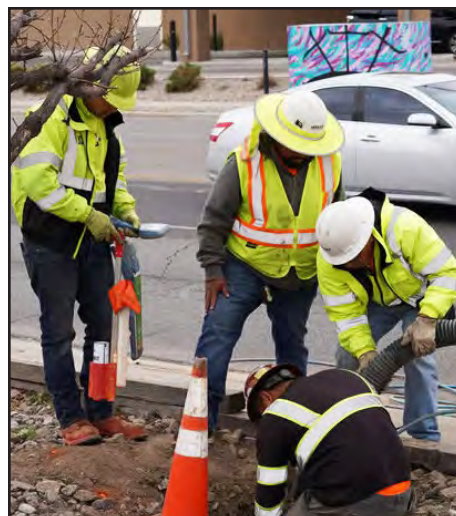
COURTESY PHOTO BY VEXUS FIBER Workers with Vexus Fiber crews install fiber optic cable for high-speed internet service in Las Cruces in February.
