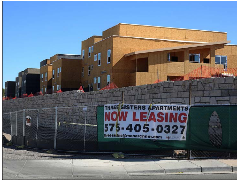
Construction continues on Oct. 28, 2024, on one of the city's affordable housing projects near the Hadley and Walnut intersection.
