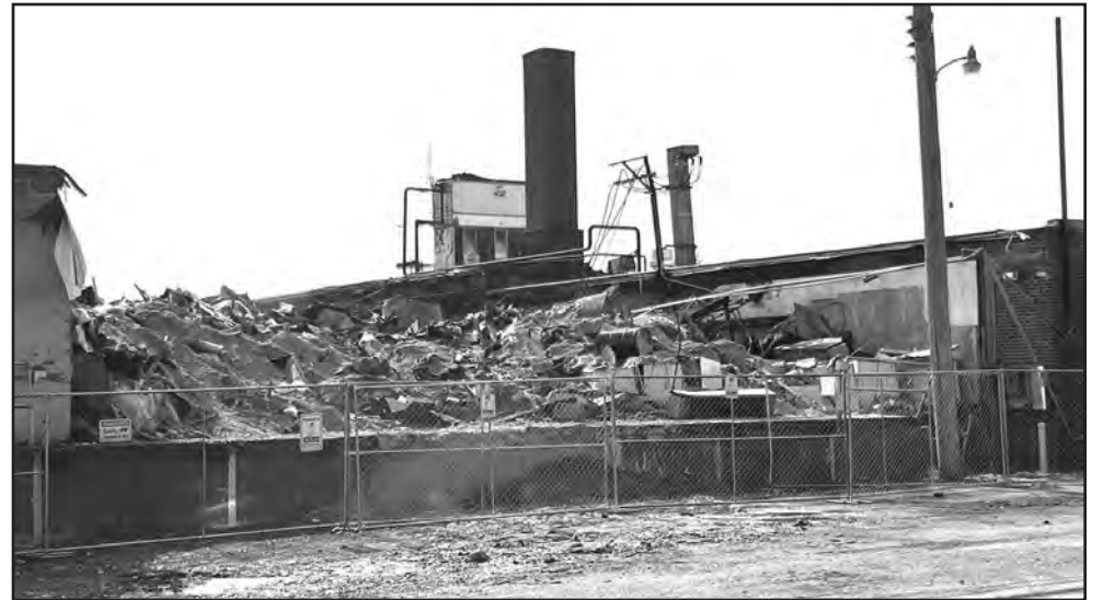
The City of Hastings has cited the Hastings Creamery after clean-up ordered to be done by Feb. 9 hasn't been in a timely fashion. The Hastings Creamery was destroyed by fire in September after closing permanently a month prior.
