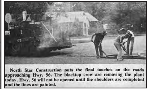
Workers are busy working on Highway 56, south of West Concord. Completion of the project is tentatively set for mid-July. The West Concord area is quite anxious for the completion of the project. Hopefully the weather will permit the construction workers to stay on schedule.
