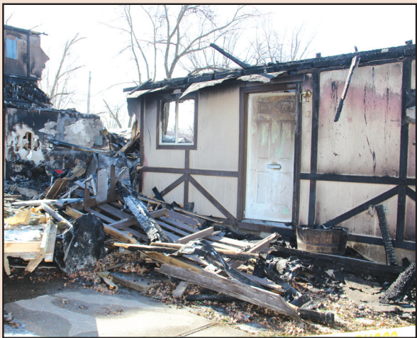
Fire damage in the 1200 block of West Breckenridge.
