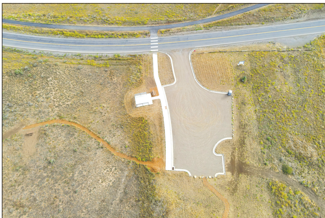
Above is the start of Phase One of the parking lot. Construction began on this portion in 2018.
