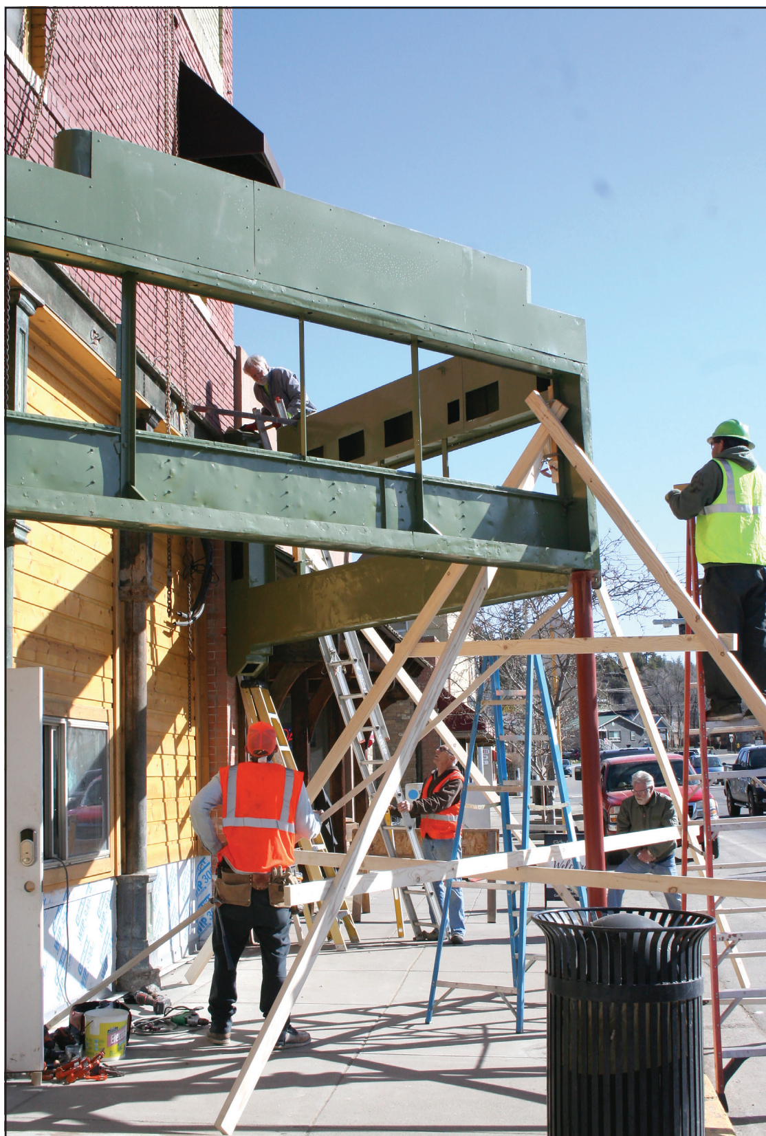
Workers install the refurbished and repainted marquee at the Liberty Theater Friday. The theater has been said to be the fourth oldest cinema in the state. Co-owner of the establishment Sherry Phillips stated last week, "We have to keep history here." It is hoped that the theater will open in mid to late summer.
