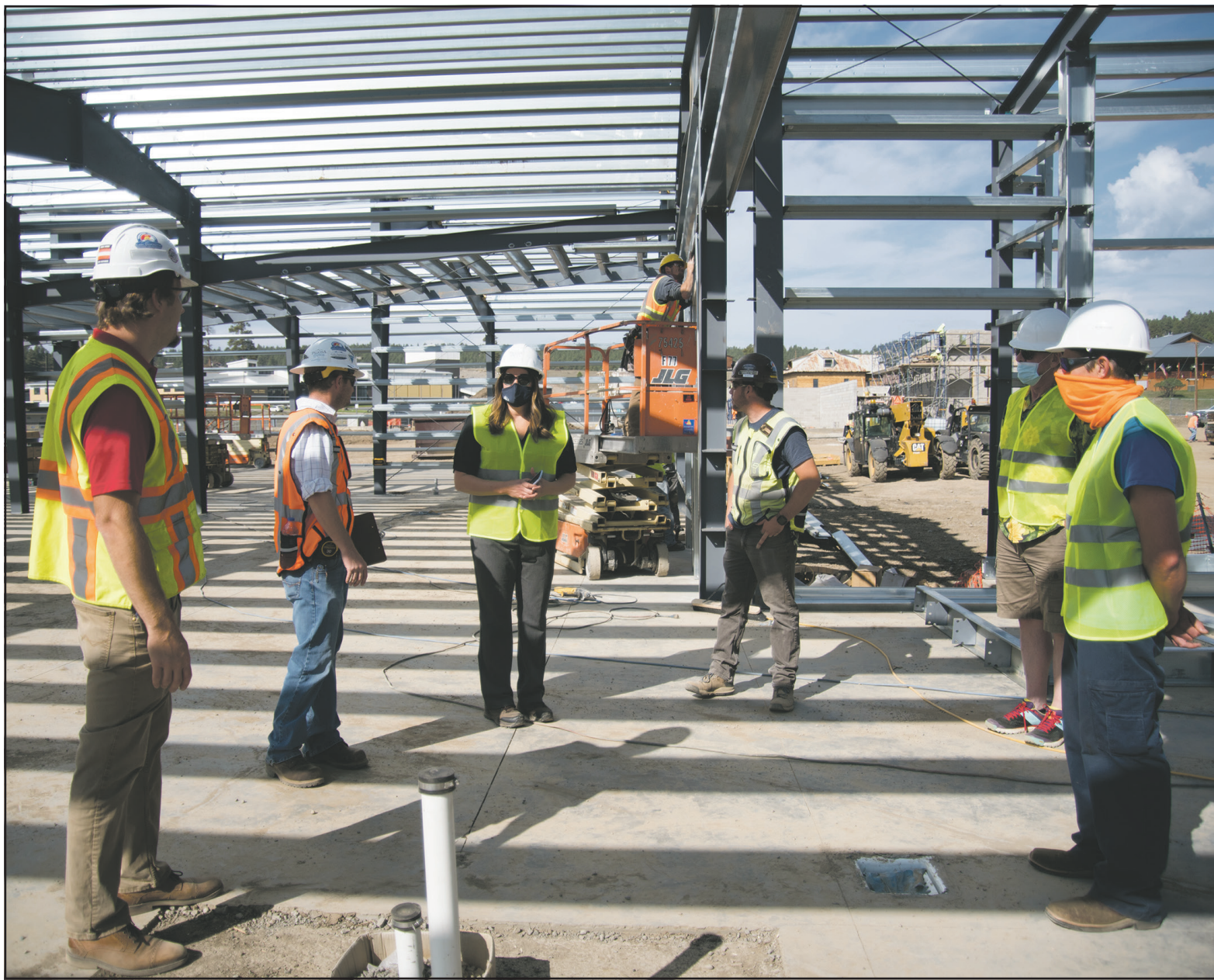
Town staff and Alcon Construction representatives led a pair of progress tours at the site of the town's new consolidated maintenance facility. The tours were attended by town employees, members of the town council and other town boards, and members of the public.
