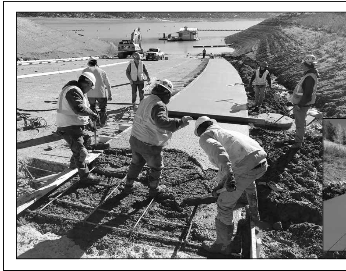
Photos courtesy Colorado Parks and Wildlife Workers at Navajo State Park pour new concrete to repair the boat ramp recently. The work should be done by late January — in plenty of time for the 2019 boating season.
