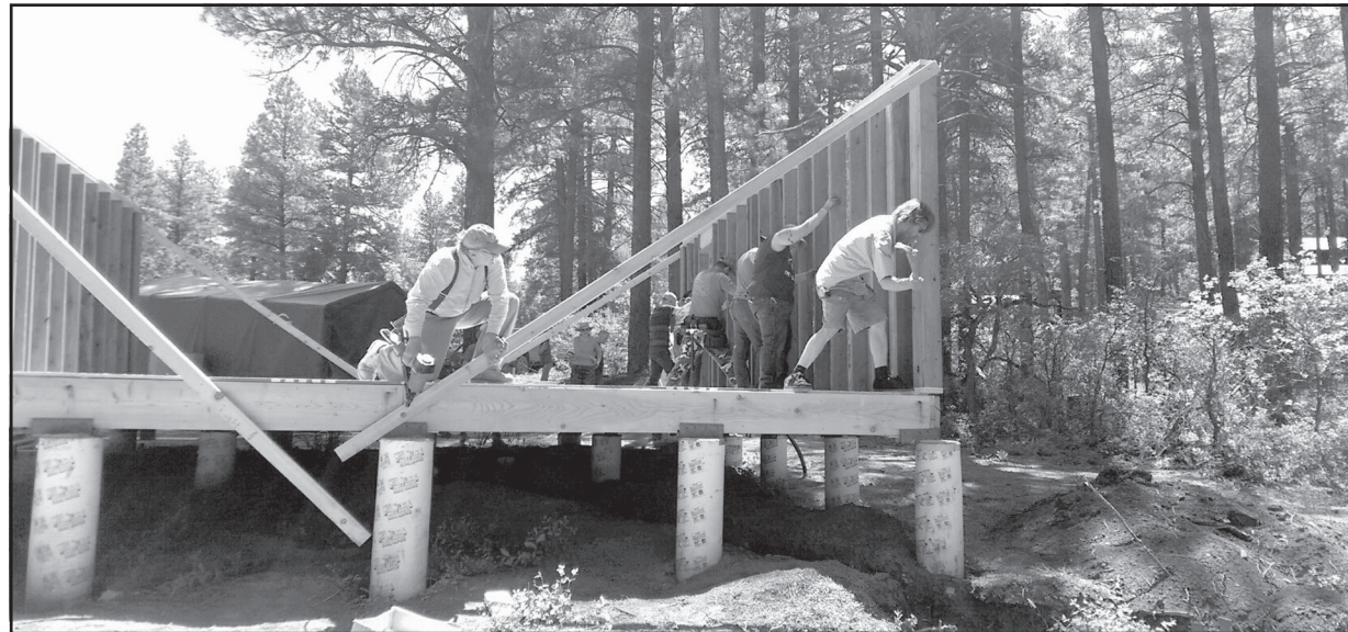
Volunteers for Starter Homes for Archuleta participate in workdays recently for a community-build home. Prior to winter, the septic system, water cistern and foundation was put in.
