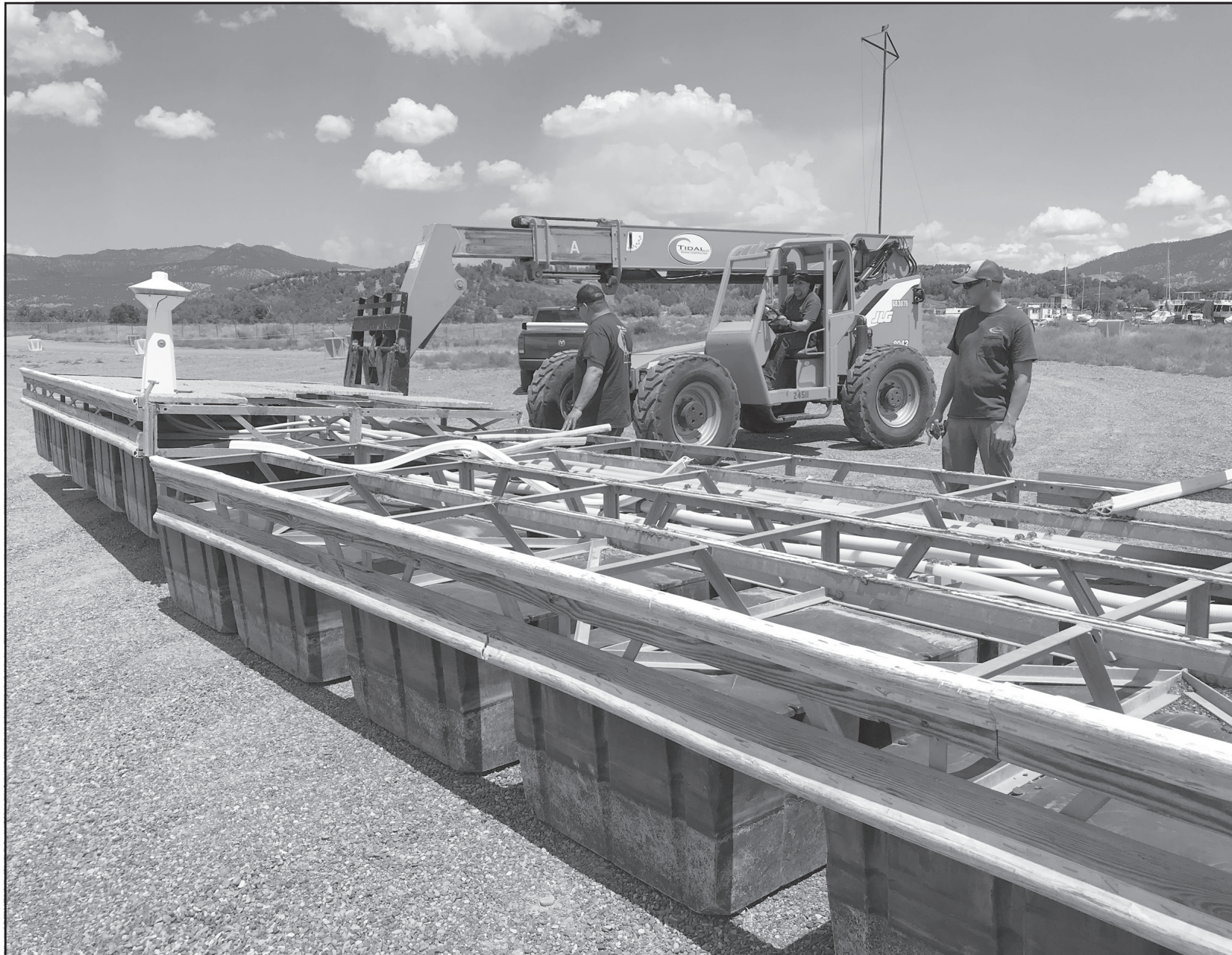
Photo courtesy Colorado Parks and Wildlife Workers begin to restore marina facilities at the boat ramp at Navajo State Park. The dock, boat slips, store and utility lines were removed earlier this year. Construction crews will reconnect the infrastructure and, if all goes as planned, the work will be completed by Labor Day.
