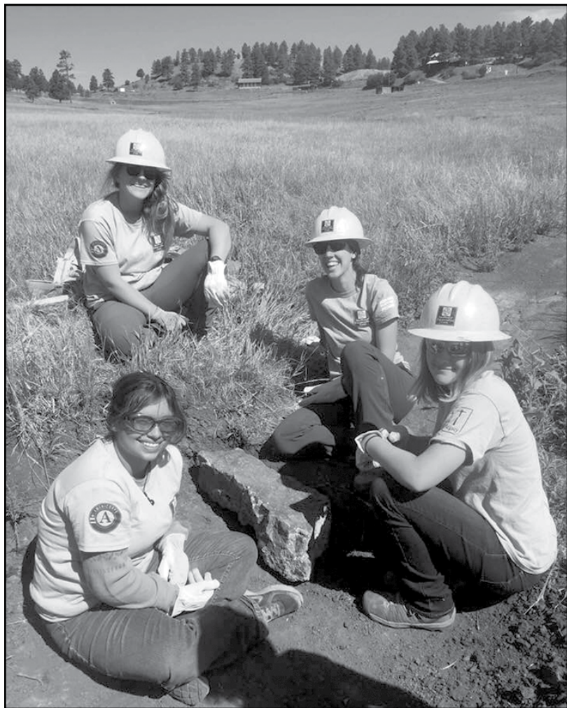
The Southwest Conservation Corp works to install four more armored crossings on the Dakota Springs Trail located behind Pagosa Springs High School the week of July 16. The crossings will ensure proper drainage along the trail.
